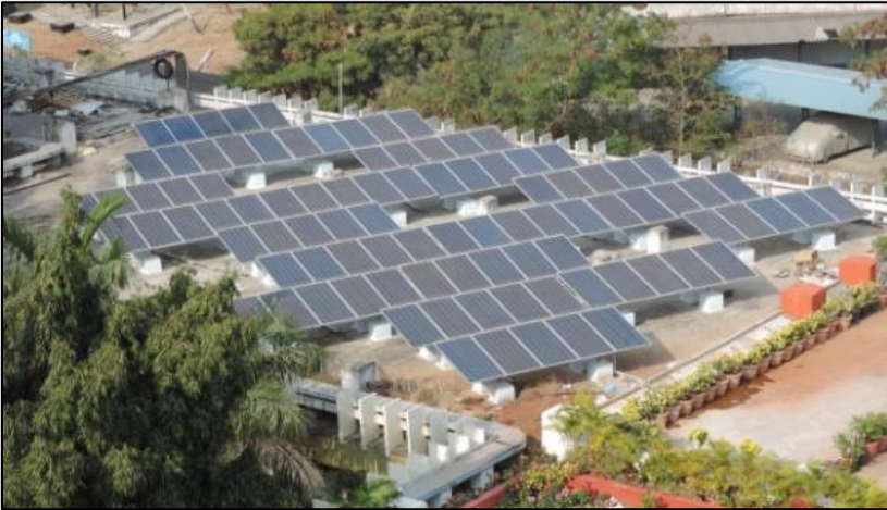
Rooftop Solar Plant
