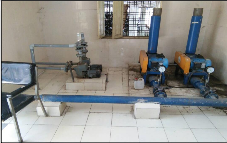
Recycling of Water & STP
